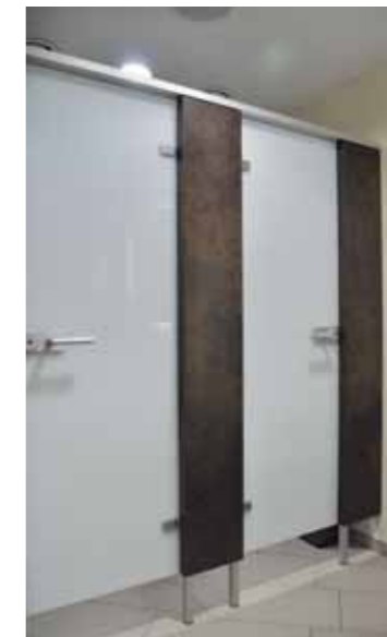
Mapet, Rottenburg Toilet cubicles and wall cladding in HPL-Compact Patina decor, glass doors and privacy screens.
